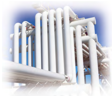
Industrial Gases Pipeline
