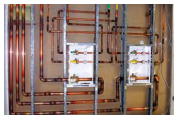
Medical Gas Pipeline
